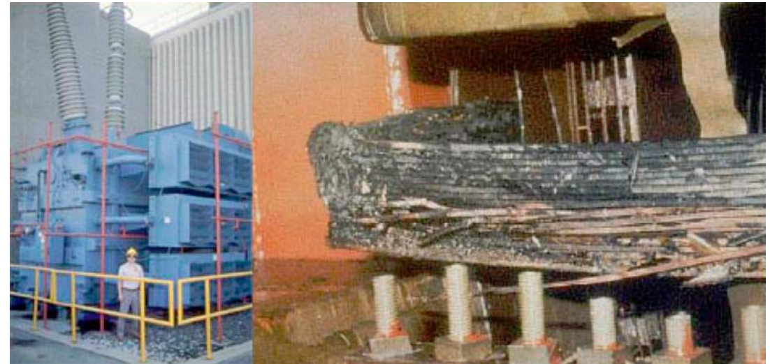
Damage to EHV transformer in New Jersey, USA.
